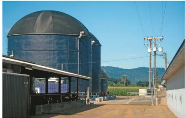
Digesters with BIOFLEX pipe installed at the Lochmead Farm
