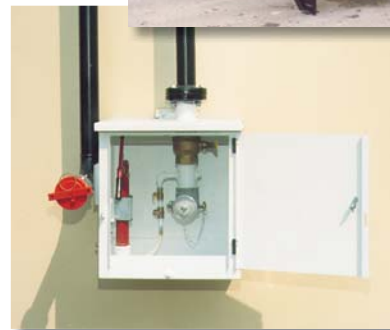
Ground Level Spill Box
