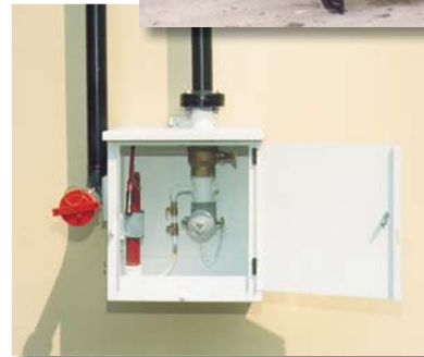
Ground Level Spill Box
