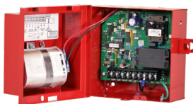
Capacitor in IQ Control Box 008800581
