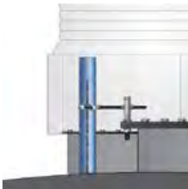
Sensor installed in bracket
